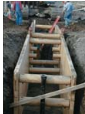
An example of a trench box with a ladder to provide a safe entry for the employee. Note: the wood cross brace at the near end of the box prevents access to the unprotected area of the trench.
